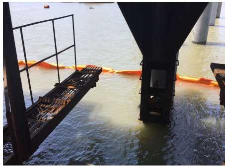
Oil containment boom deployed on-site to protect the favourable environment for pacific oysters farming in Long Son Commune.
