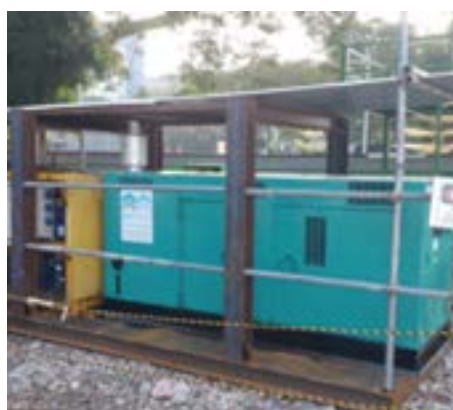
Good Housekeeping on Site – Gen Set and welding equipment cage discourages unwanted meddling to equipment.
